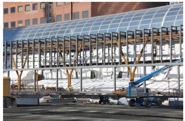
View of the “Y” column installation at the UP Express station inside the Skywalk
