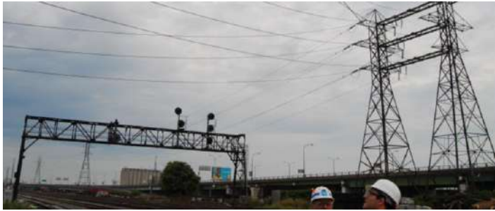
Figure 9-1 Hydro One Transmission Lines at UP Express Corridor (Milepost 0.7)
