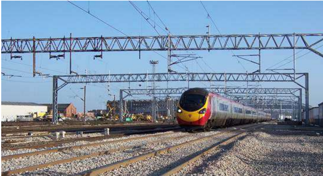
Figure 1-2. Example of OCS Support Structures (Portals)
