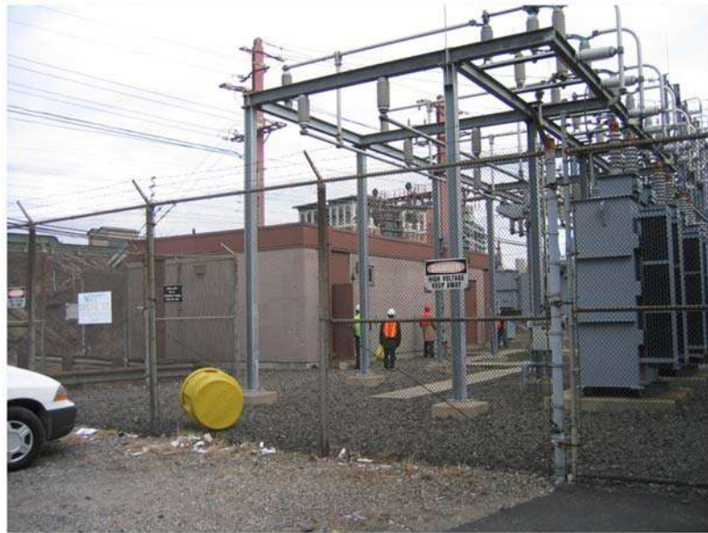
Figure 1-3. Typical Paralleling Station
